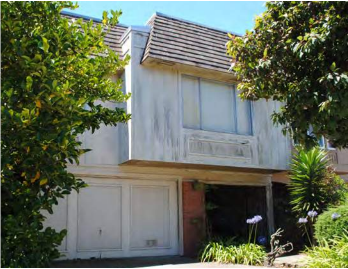
[5-21] 244 Gold Mine Drive | This Galli house has high integrity, despite its poor condition. The siding, windows, garage door, light fixture, shingles, and house numbers are all original. [Hannah Simonson]
