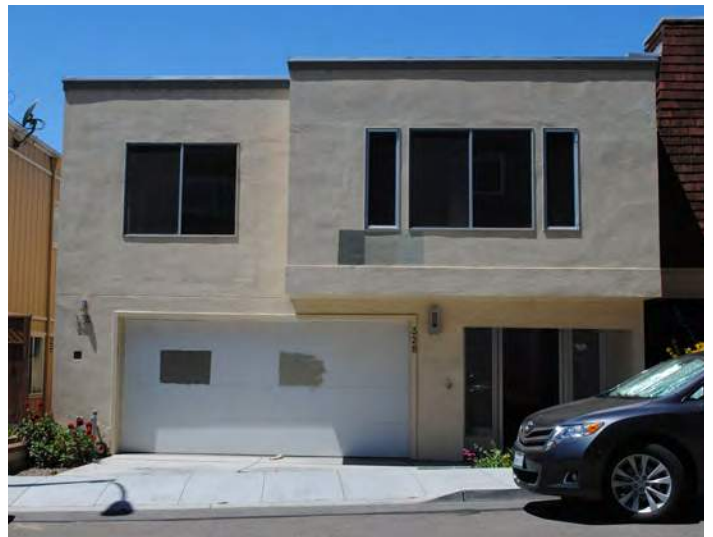
[5-24] 328 Gold Mine Drive | The character-defining Neo-Mansard roof of this Galli home has been removed. Without the single-most important feature, this home has no integrity and would be a non-contributor in any potential district. [Hannah Simonson]
